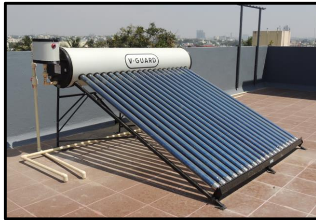
Figure 1.1 Solar water heater for domestic purposes
